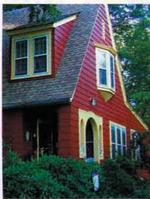
Attentive repair of the oriel window and arched entry made this Tudor a shoe-in for a nomination.
